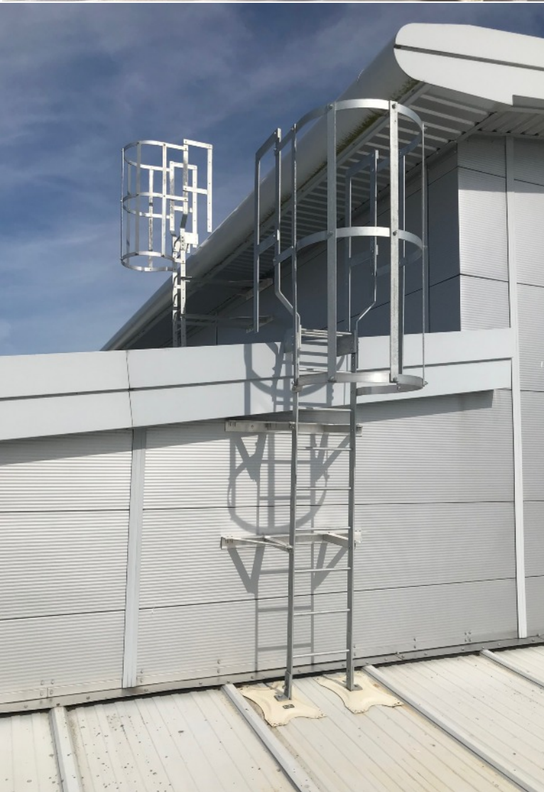
A sample of Access Ladders supplied and installed by our engineers.
